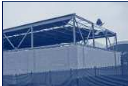
The new athletic facility is currently under construction on South Ithan Avenue.
